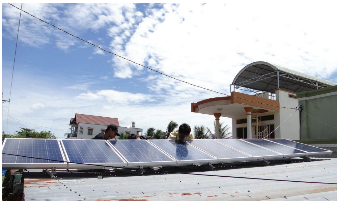
Fostering rural electrification with renewable energy. © GreenID
